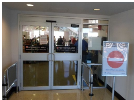
Figure 16: Sensor Activated Doors
