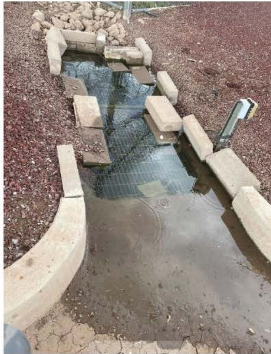
Exhibit 1. Blocked Bio-Swale Drainage Pipe and standing water between the parking lot and main security entrance at CCCC, as OIDO observed on August 11, 2022.
