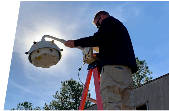
The SDS Outdoor gunshot detection technology is quickly installed for field assessment. Photo: S&T
