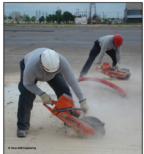
Figure 1. SMEs cut airport runway concrete using multipurpose cutoff saws and test blades.
