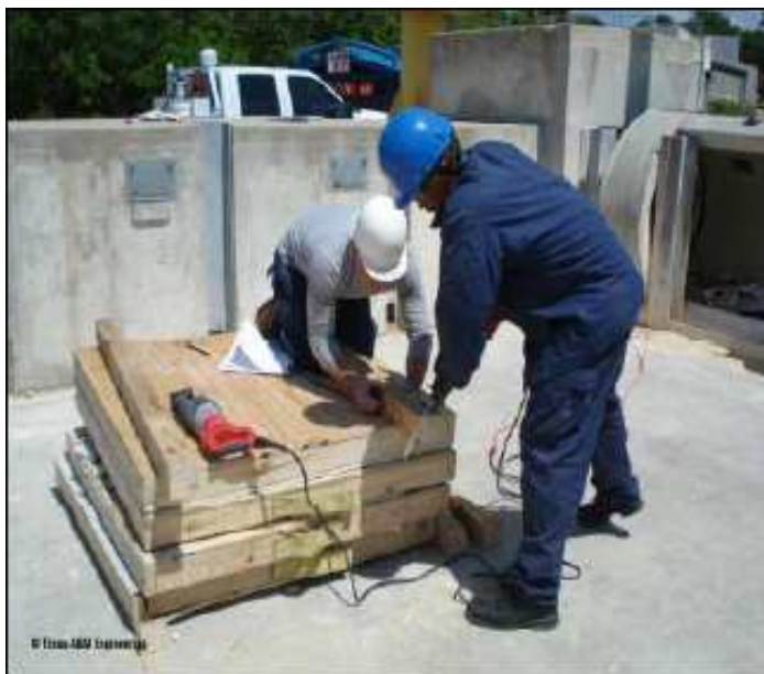
Figure 2. An emergency responder SME cuts 4x4 structural cribbing using multi-purpose reciprocating saw blades.
