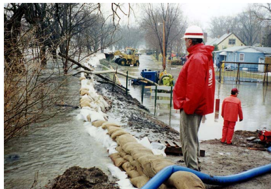
Portable and Mobile Pumps are Used for Flood Response in Granite Falls, Minnesota
