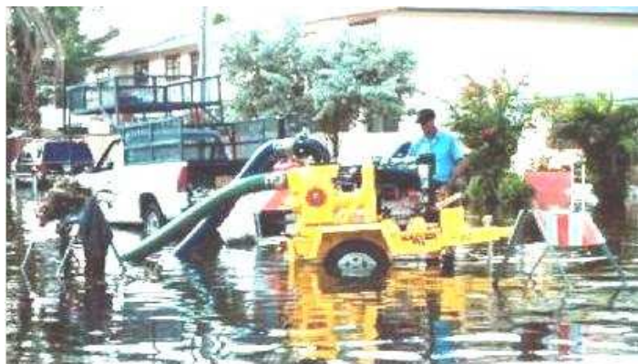
A trailer-mounted trash pump is used for flood recovery in Sweetwater, Florida (Kevin Galvin/FEMA News Photo)
