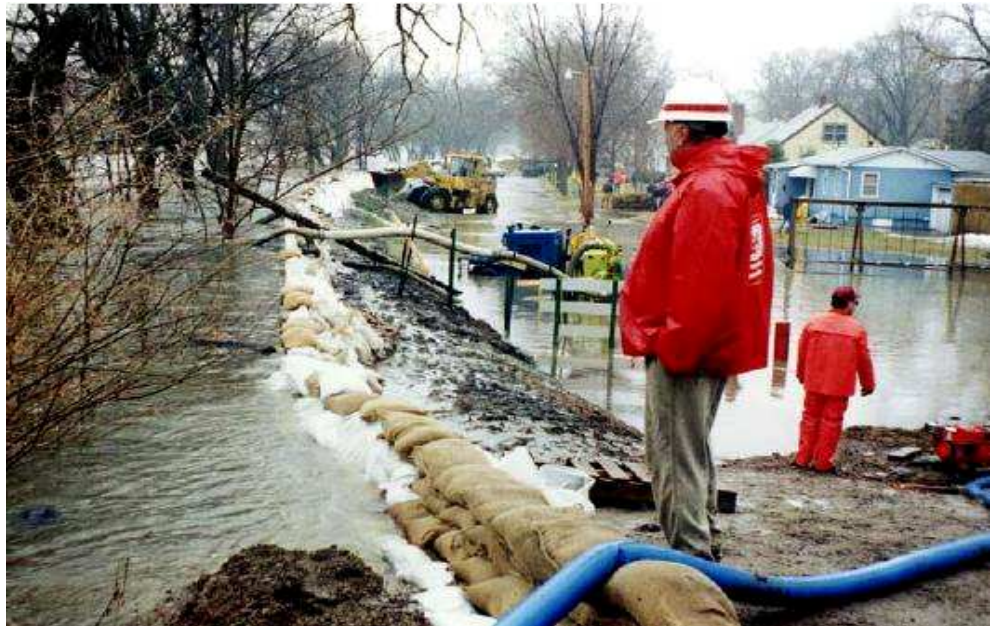
Portable and mobile pumps are used for flood response in Granite Falls, Minnesota
