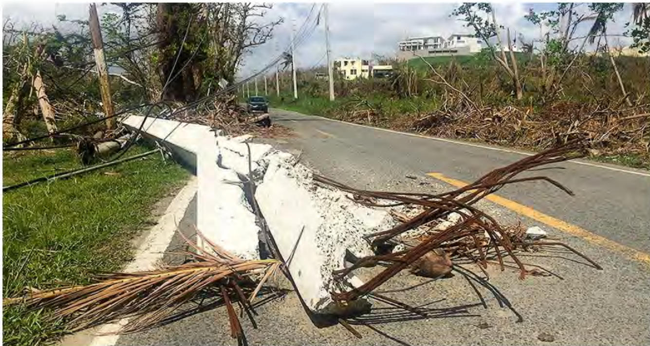
A shattered concrete power line blocked traffic yesterday outside of Naguabo, on Puerto Rico's east coast. Almost three weeks after Hurricane Maria, restoration of the electric grid has barely begun. David Ferris/E&E News
