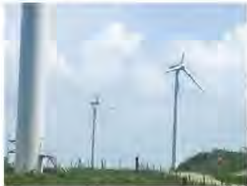
The gusts of Hurricane Maria snapped turbine blades at the 23-megawatt Punta Lima wind farm in Puerto Rico. David Ferris/E&E News
