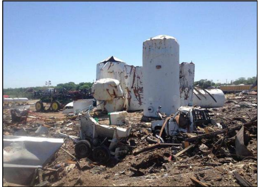
Damaged volumetric tanks and equipment at the Adair Grain Inc. Fertilizer Plant in West, Texas. (Photo courtesy of the Environmental Protection Agency (EPA); EPA website )
