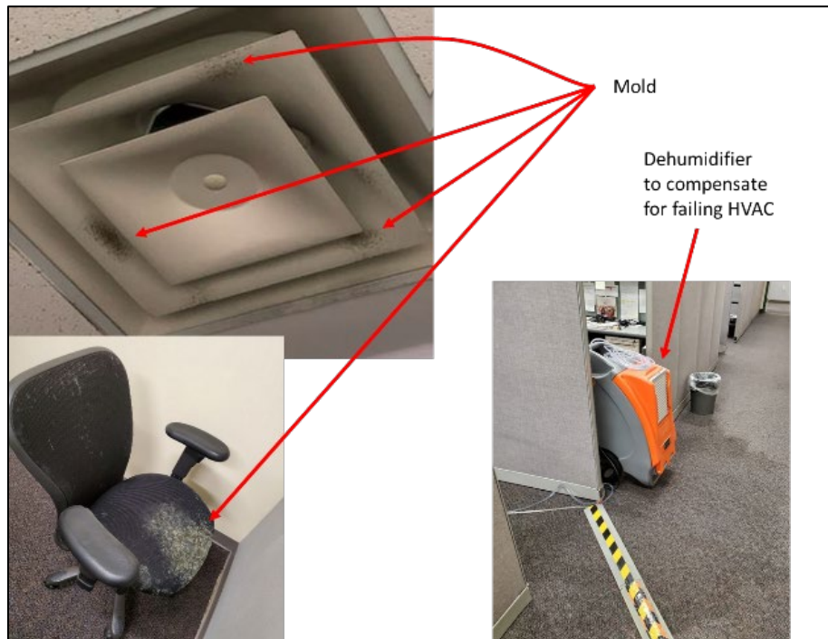
Figure 2-4. Failing HVAC systems and overcrowded areas have resulted in mold growth in the office area.
