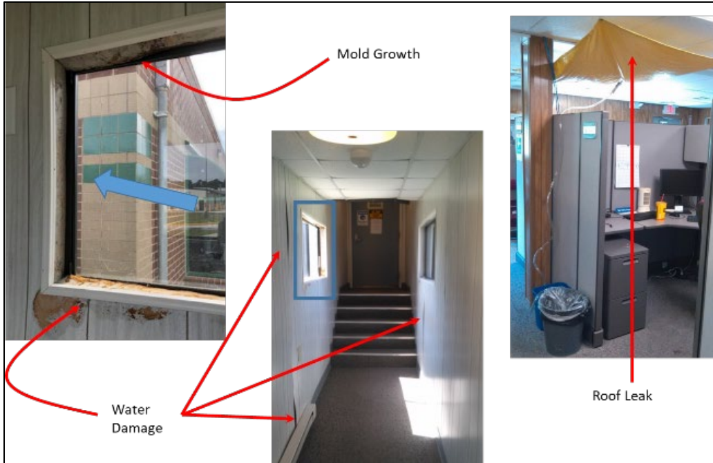
Figure 4-3. Temporary buildings have exceeded their useful life and are experiencing structural failure.
