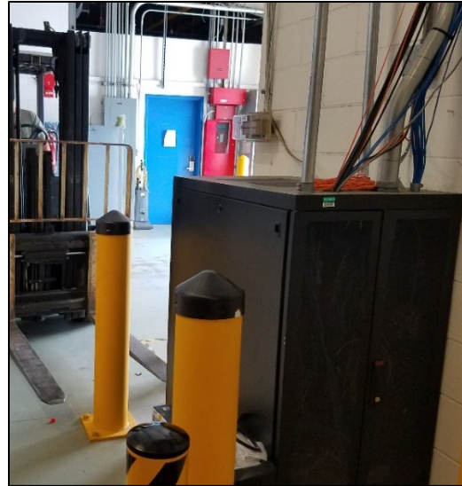
Figure 2-1. Network and IT equipment near garage entrance of TSL Building 319 without appropriate climate control
